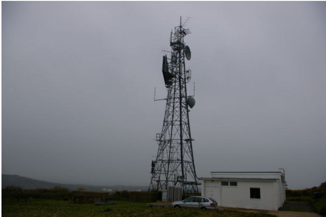
Figure 3 – The Arqiva site’s antennas are located on the actual TV transmitter
