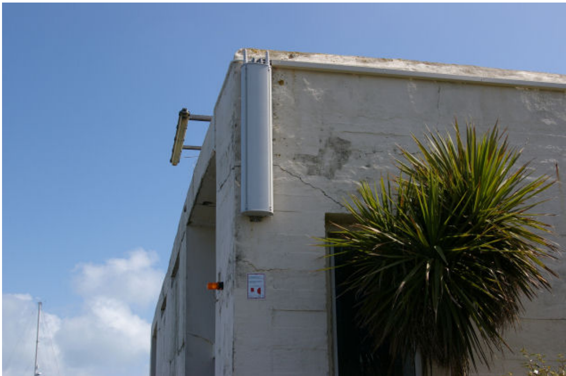
Figure 4 – Detail of the antenna installation
