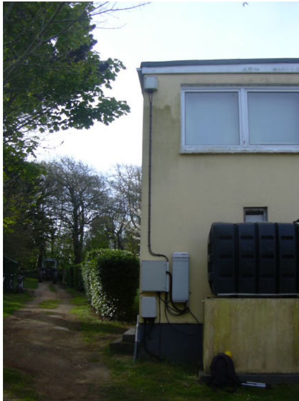
Figure 3 – The wall-mounted antennas at La Moinerie
