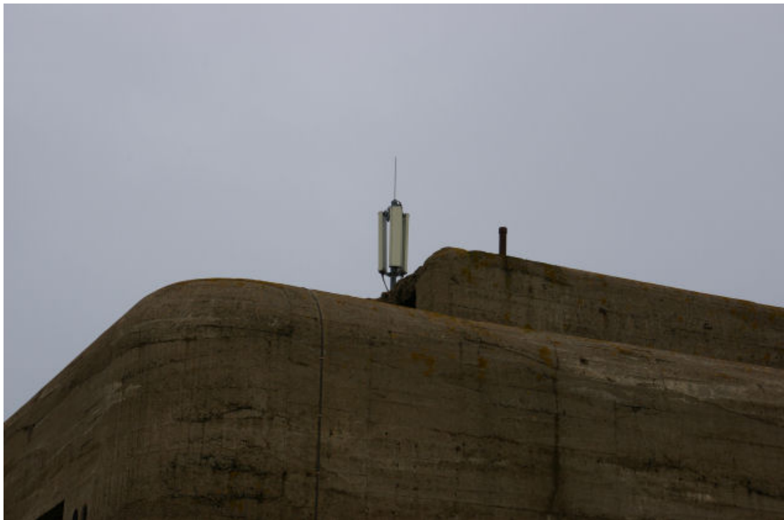
Figure 4 – Antennas on the roof top
