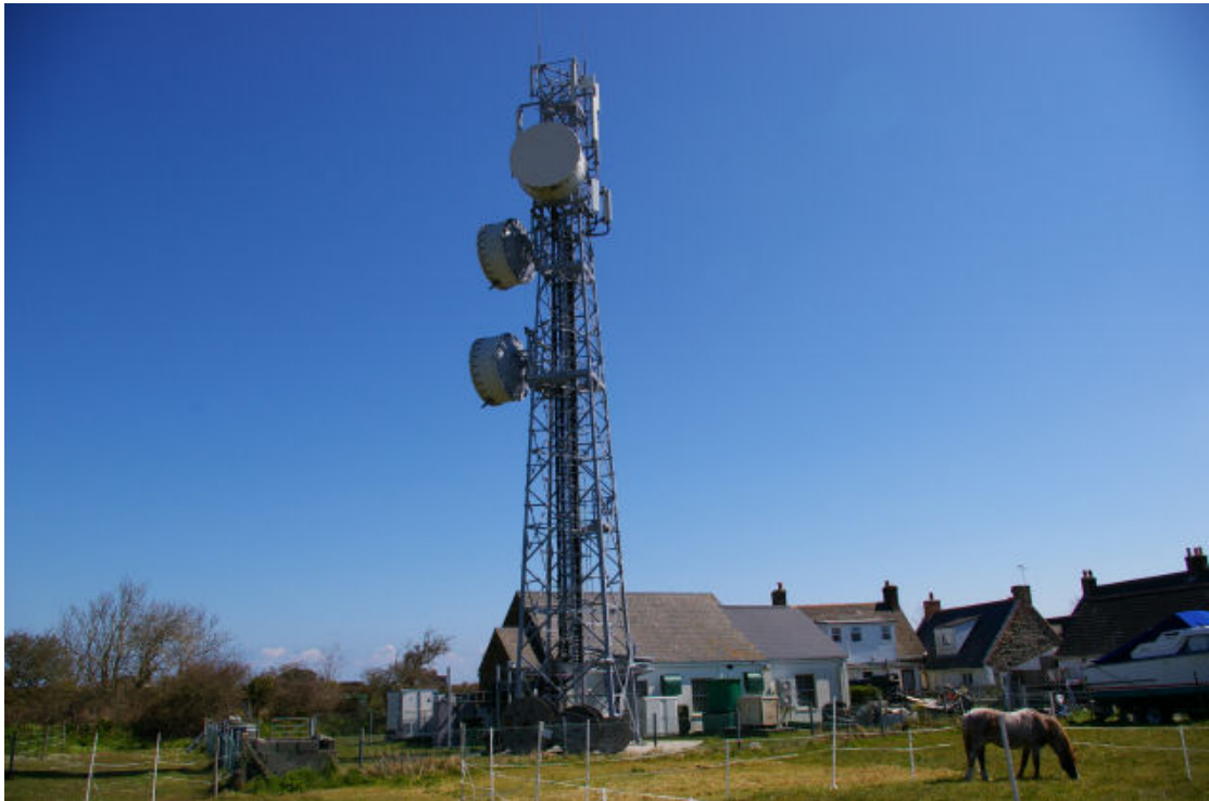
Figure 3 – Existing Mast at Sark T.E.
