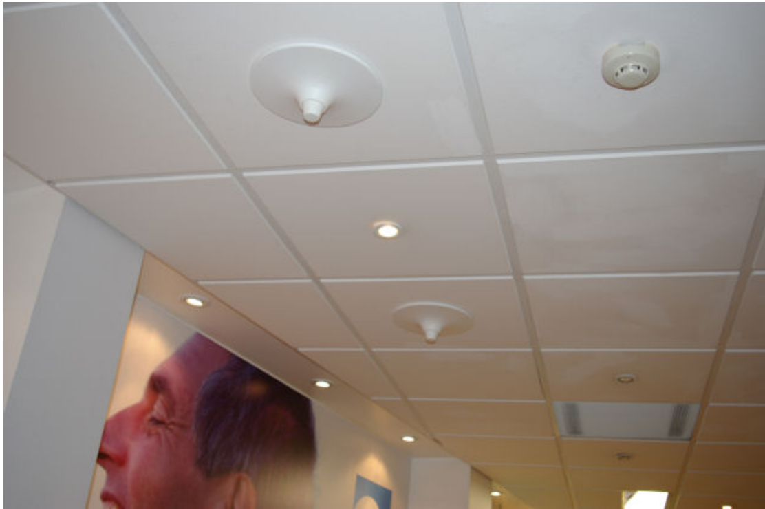
Figure 3 – Antenna Installations on the ceiling
