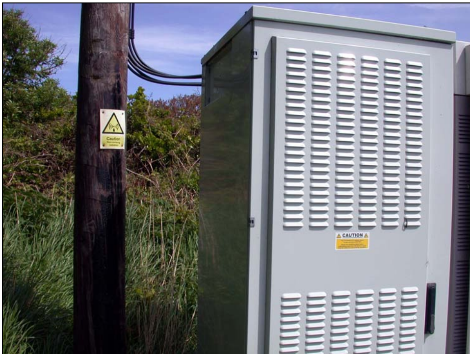
Figure 4 - Existing Installation with radiation hazard sign on the pole
