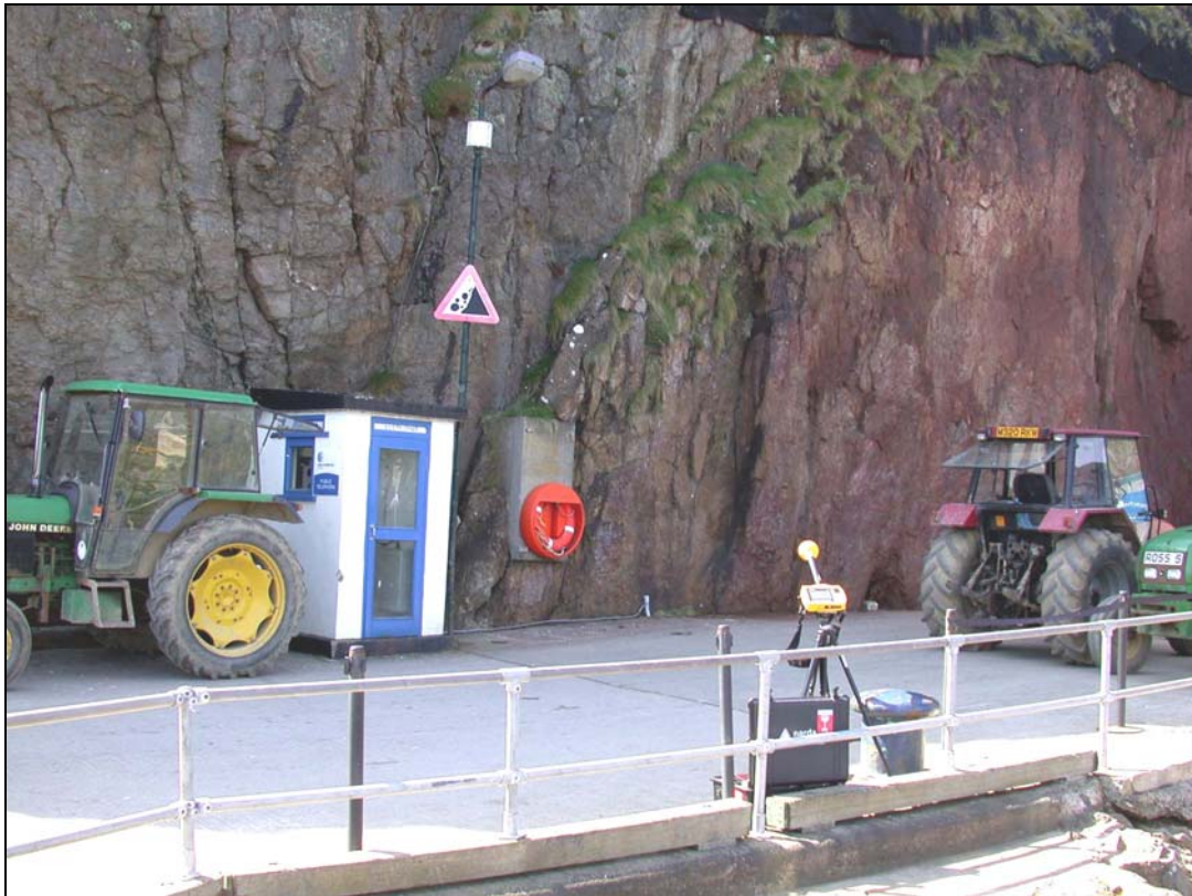
Figure 3 – View of the antenna attached to the top of the lamp post and the spectrum scan location (Test Site)
